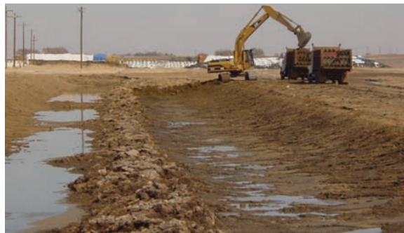
Figure 3. Gravitational solids separation basin during clean out. The water enters the basin in the foreground and slows to allow solids to separate from the water, which continues to flow through the basin and to the lagoon.
